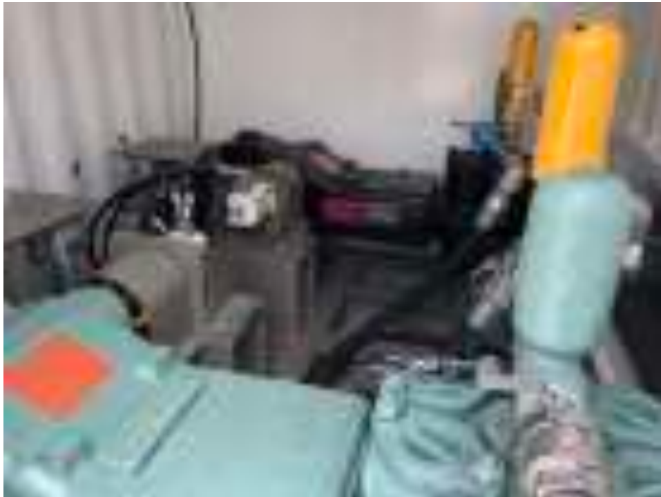
Mud pumps in covered housing
