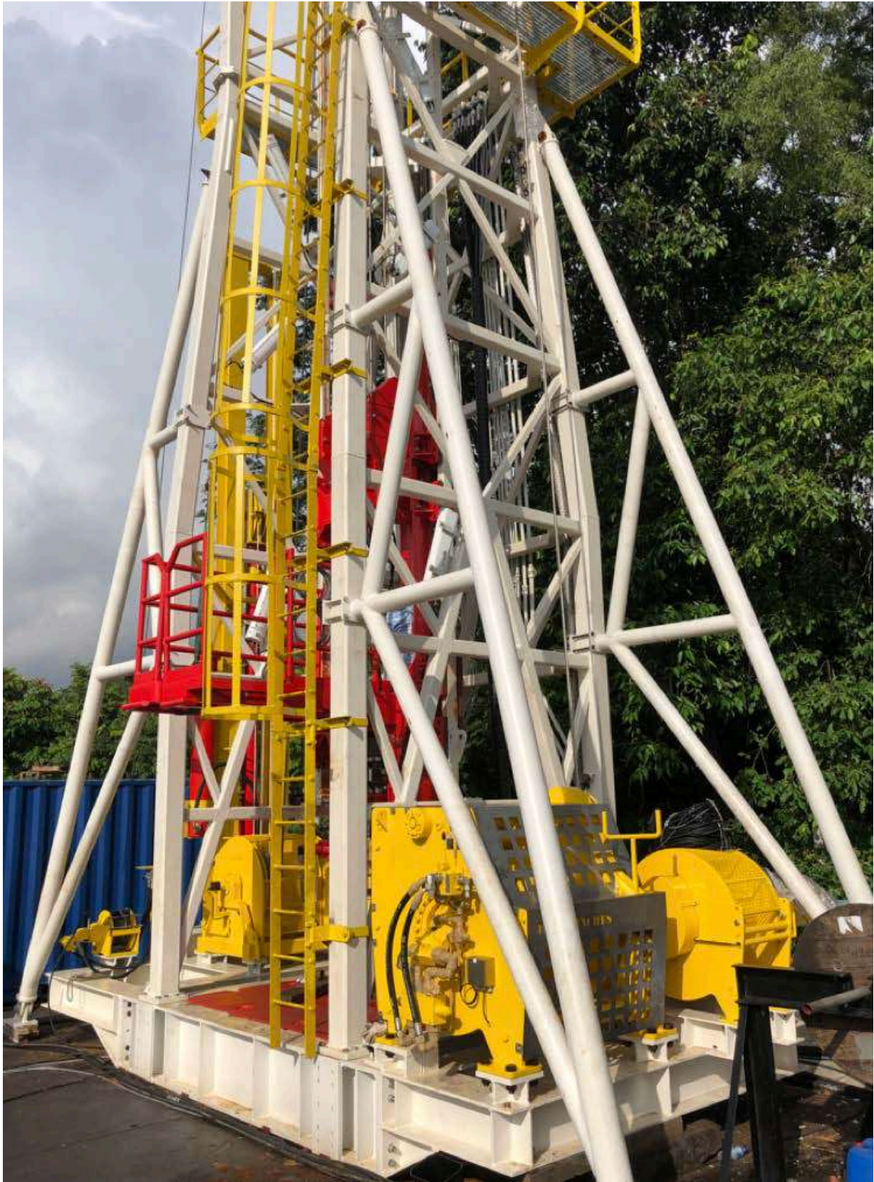
Lower derrick mast, braces and base frame with installed winches
